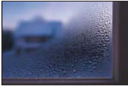
Condensation on the inside of a windowpane.
